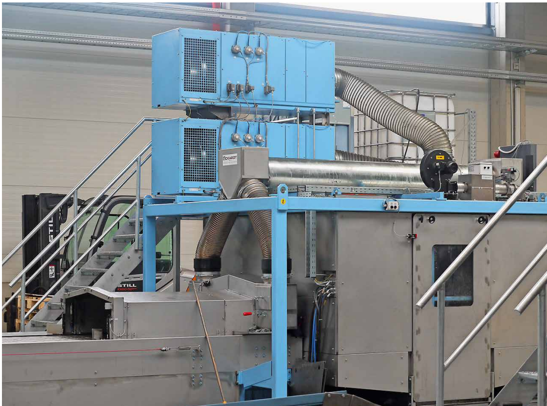
Side view of the system with the discernible filter system on top.
